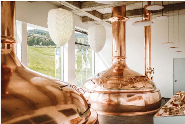
Image 1: Tip-top inside and out: The old Huppmann brewhouse held up for nearly 60 years before Huppmann's successor GEA refurbished everything under the gorgeous copper domes in 2018. Photo: Brauerei Zötler/Petra Reger – wertvoll fotografie
